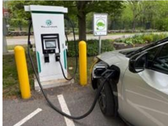
Tellus Power Green Level 3 Charging Station (the left port is the CCS1 and the right the NACS)
