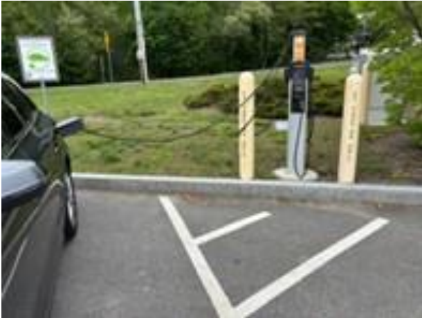
ChargePoint Level 2 Charging Station
