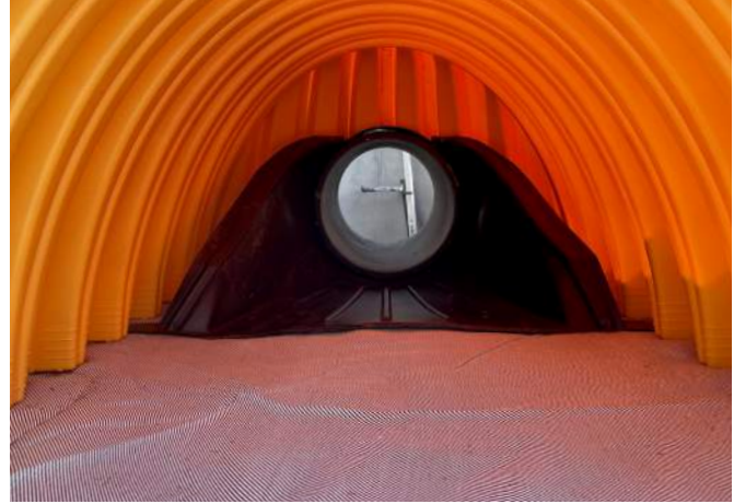
Looking down the Isolator Row PLUS
